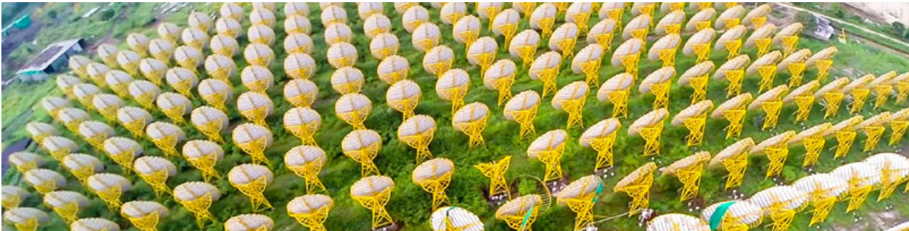
Solar Thermal Power Plant, Abu road, India. Photo Brahma Kumaris
