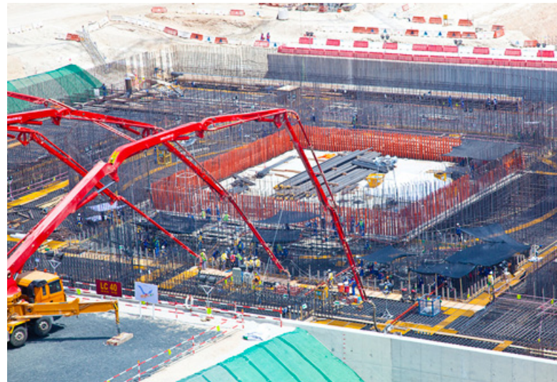
A KEPCO-led consortium is building the Barakah Nuclear Power Plant in Abu Dhabi
