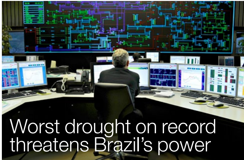
The ONS electricity grid control room for the south-eastern region of Brazil, the part of the country worst affected by the current drought. (Photo: ONS)
