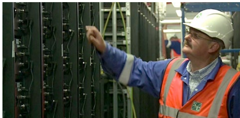
An engineer inspects batteries at Europe's largest battery storage project.
