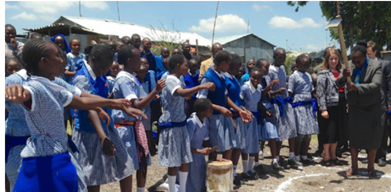
Students celebrate breaking ground on a biomass toilet project that will generate enough energy to power their school. (Photo: Rudy Gharib/USAID)
